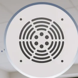
Two built-in cooling vents
