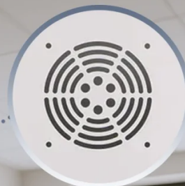
Two built-in cooling vents
